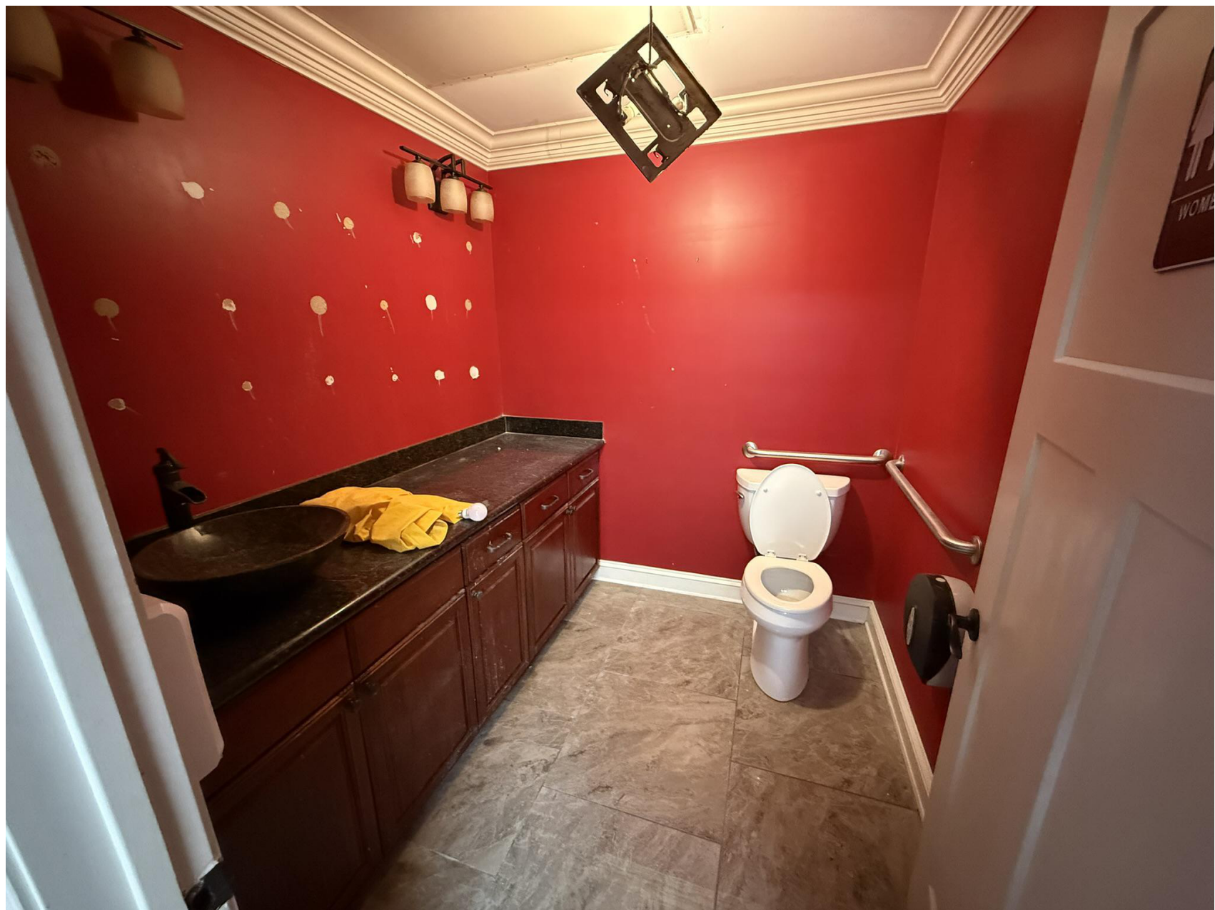
PHOTO OF EXISTING RESTROOM. DEMOLISH EXISTING CASEWORK AND SINK. REPAIR DAMAGED AND MISSING MATERIAL BEHIND CABINET. PROTECT EXISTING FINISHES THROUGHOUT CONSTRUCTION.
