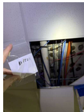
INTERIOR PIPE INSULATION/WRAP (A1-PI2-1)
