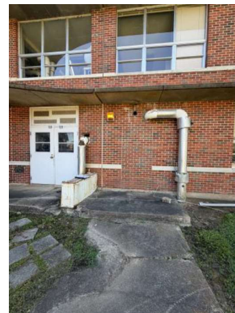
EXTERIOR INSULATED PIPES
