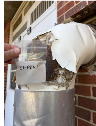
EXTERIOR PIPE INSULATION (C1-PI1-1)
