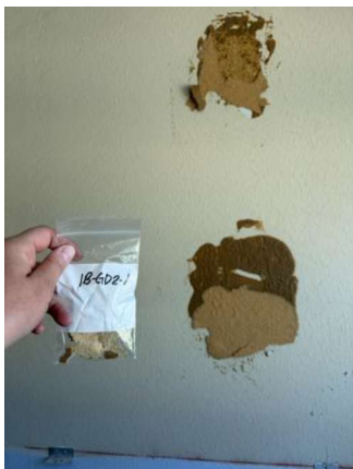
GLUE PATCH ON WALL (1B-GD2-1)
