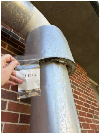
EXTERIOR PIPE INSULATION (C1-PI1-2)
