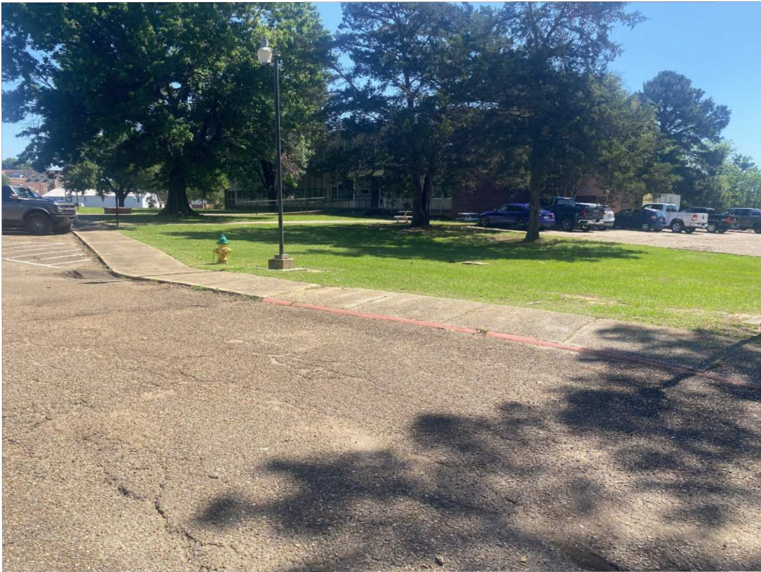
5/13/2026 FIRE HYDRANT & WATER VALVE TO PROTECT IMG_9962.jpg
