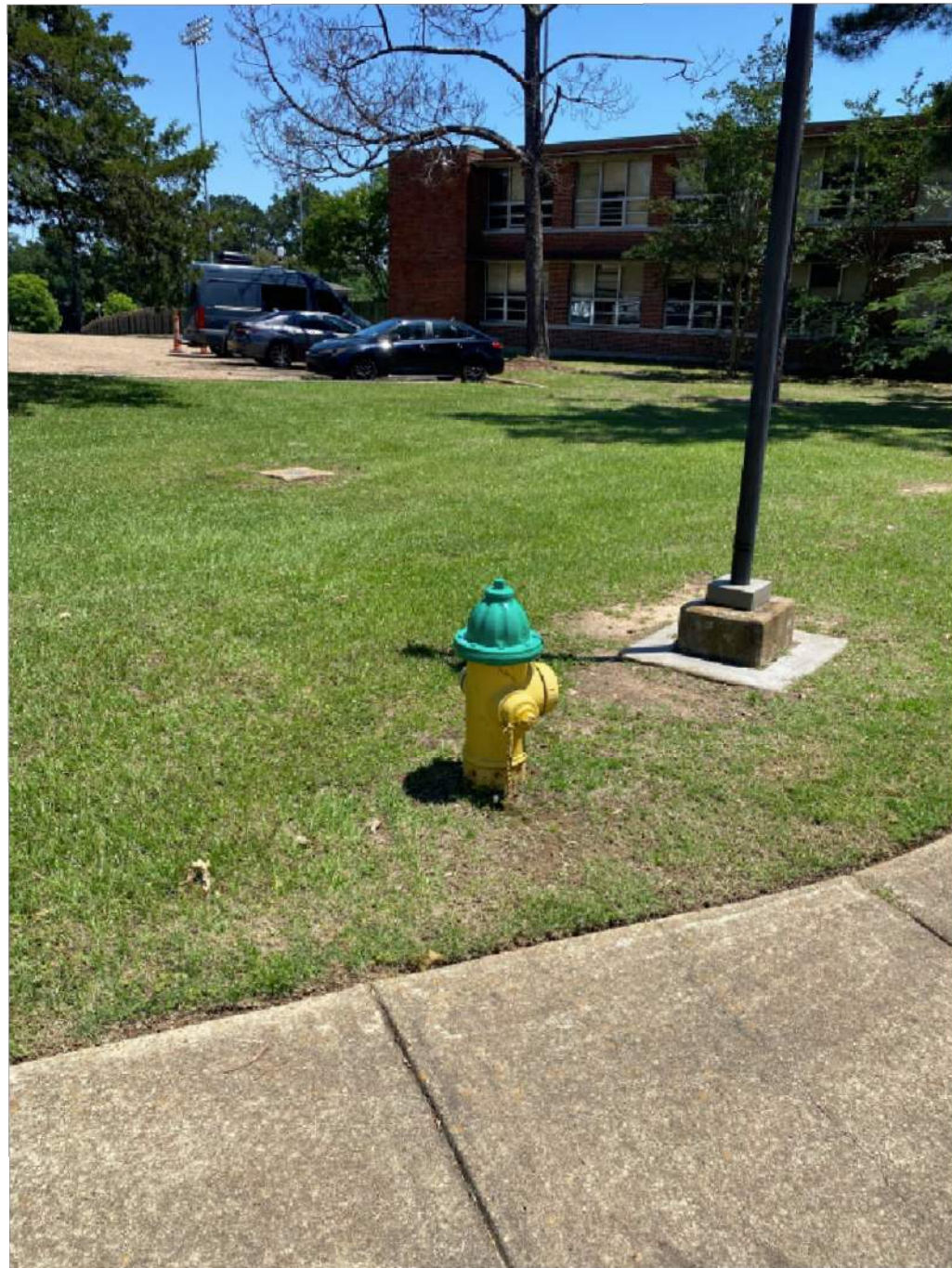
5/13/2026 FIRE HYDRANT & WATER VALVE TO PROTECT IMG_0017.jpg
