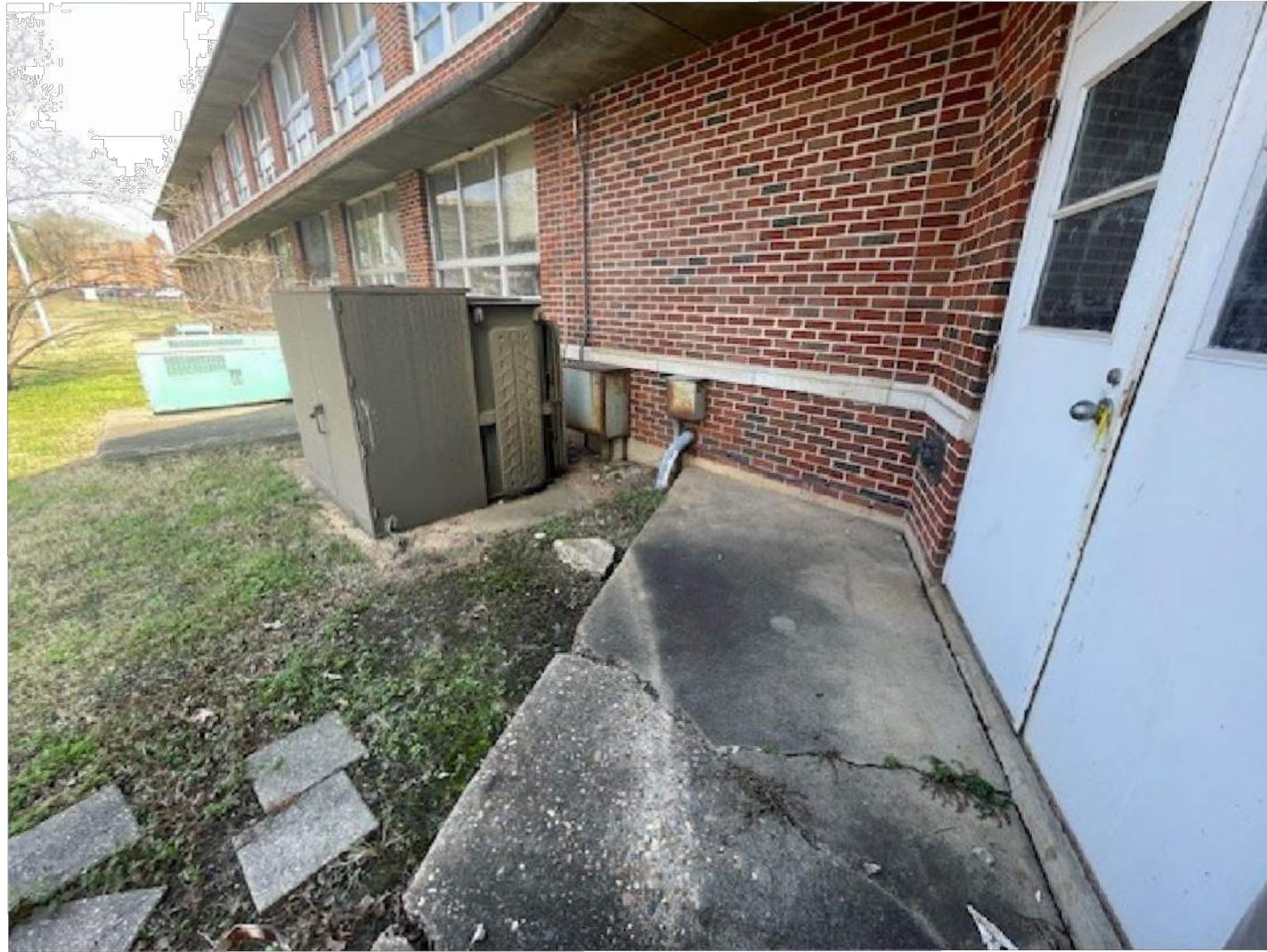
2/13/2026 TRANSFORMER & PAD TO REMAIN Photo 31.jpg
