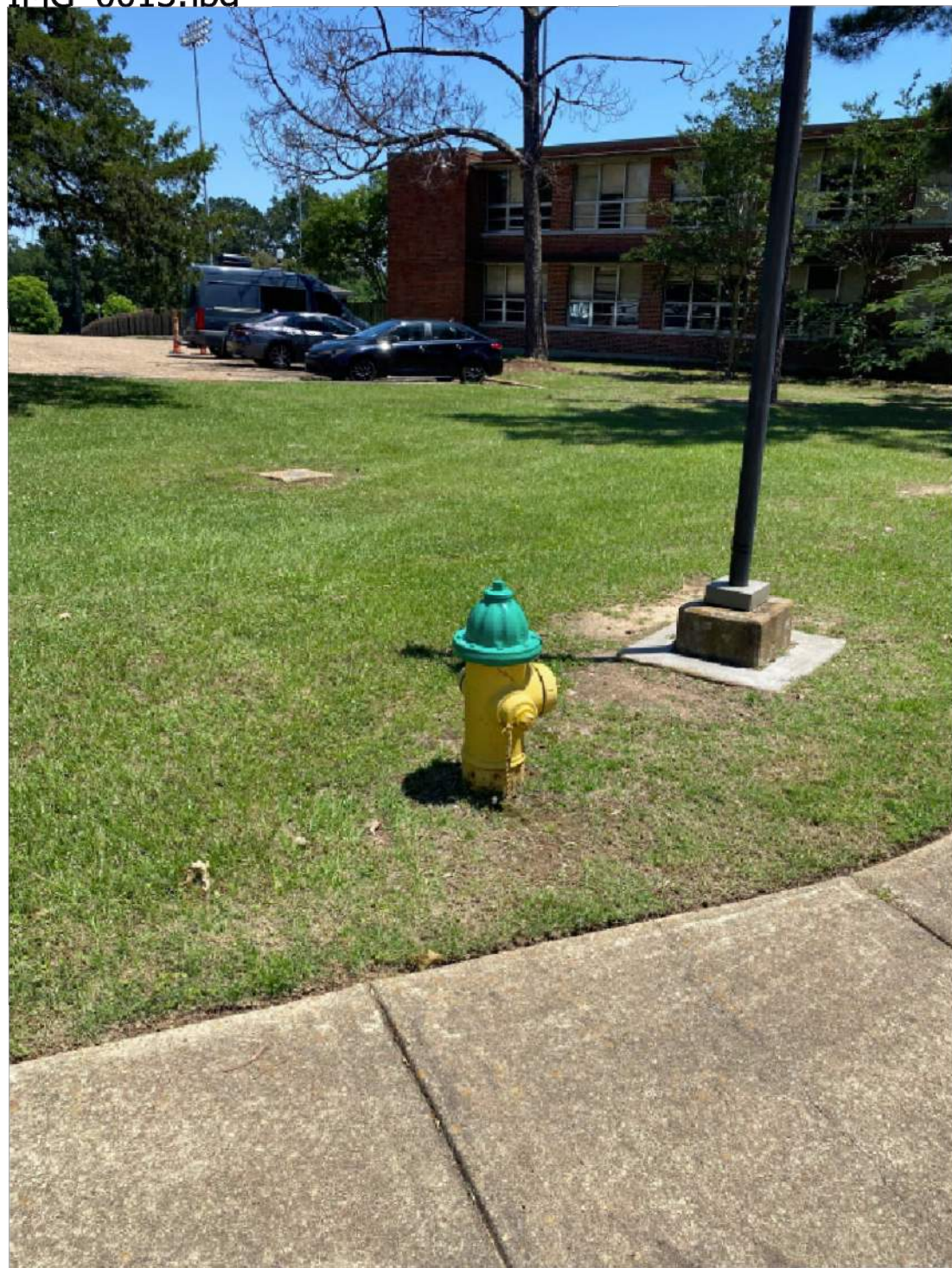
5/13/2026 FIRE HYDRANT & WATER VALVE TO PROTECT IMG_0017.jpg
