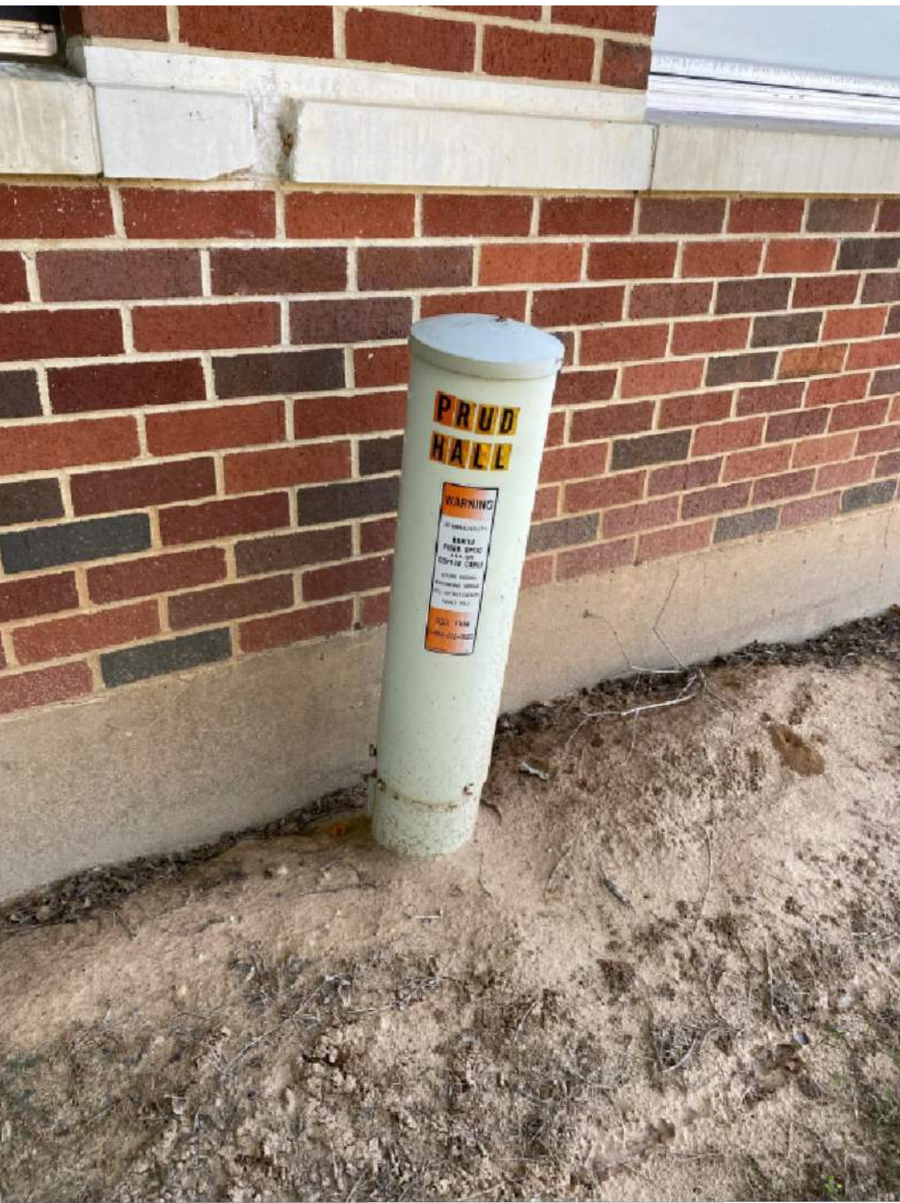
5/13/2026 TELECOM MARKER BESIDE BUILDING TO REMOVE. COORDINATE WITH THE UTILITY OWNER TO VERIFY UTILITY STATUS BEFORE DEMOLITION. IMG_9979.jpg
