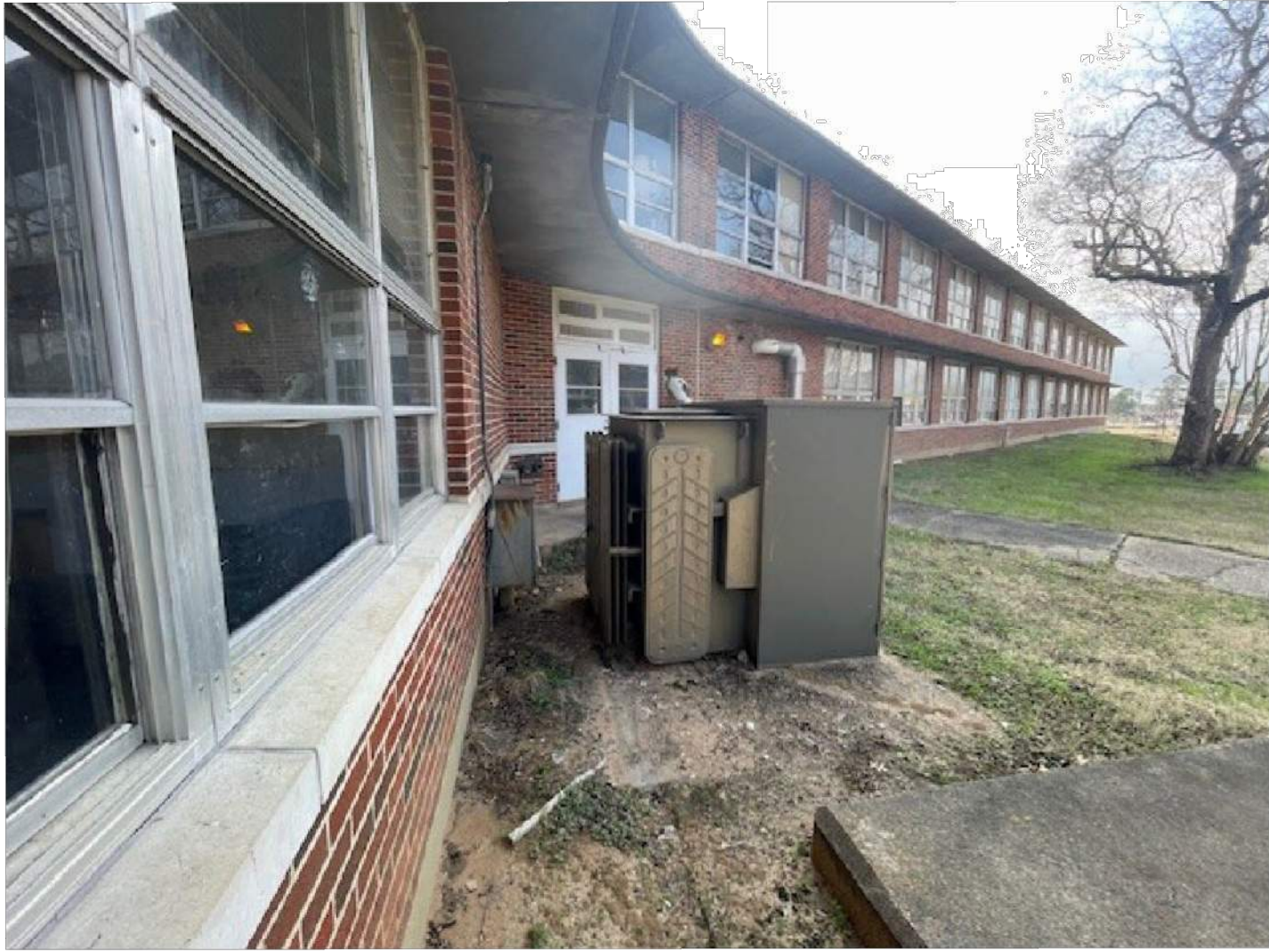
2/13/2026 TRANSFORMER & PAD TO REMAIN Photo 30.jpg
