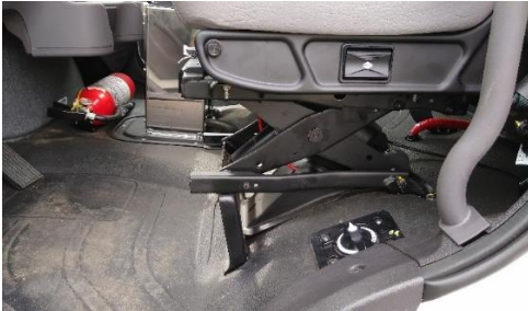
Figure 1: Battery disconnect switch location in accordance with spec.
