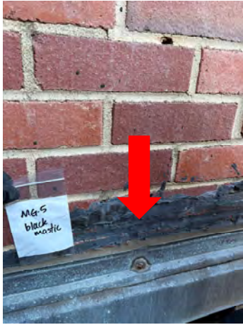
MG-5 BLACK MASTIC BEHIND FLASHING
