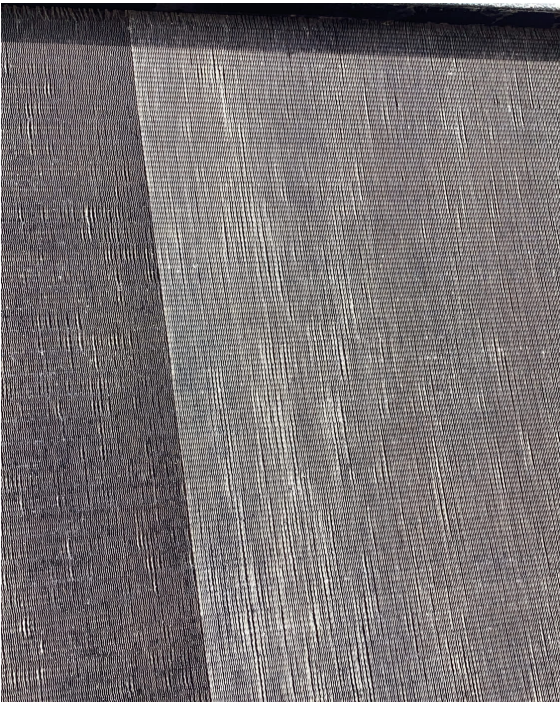
Chiller coils after cleaning.
