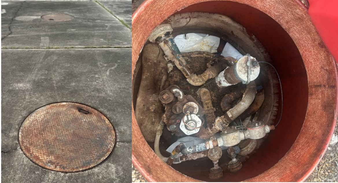
Photo of anode connected in tank
