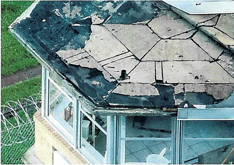
Attachment D - Pictures of Damages RFx 3000024712
