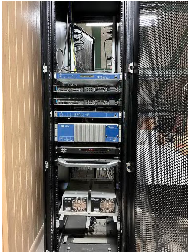
PDCS Control Cabinet
