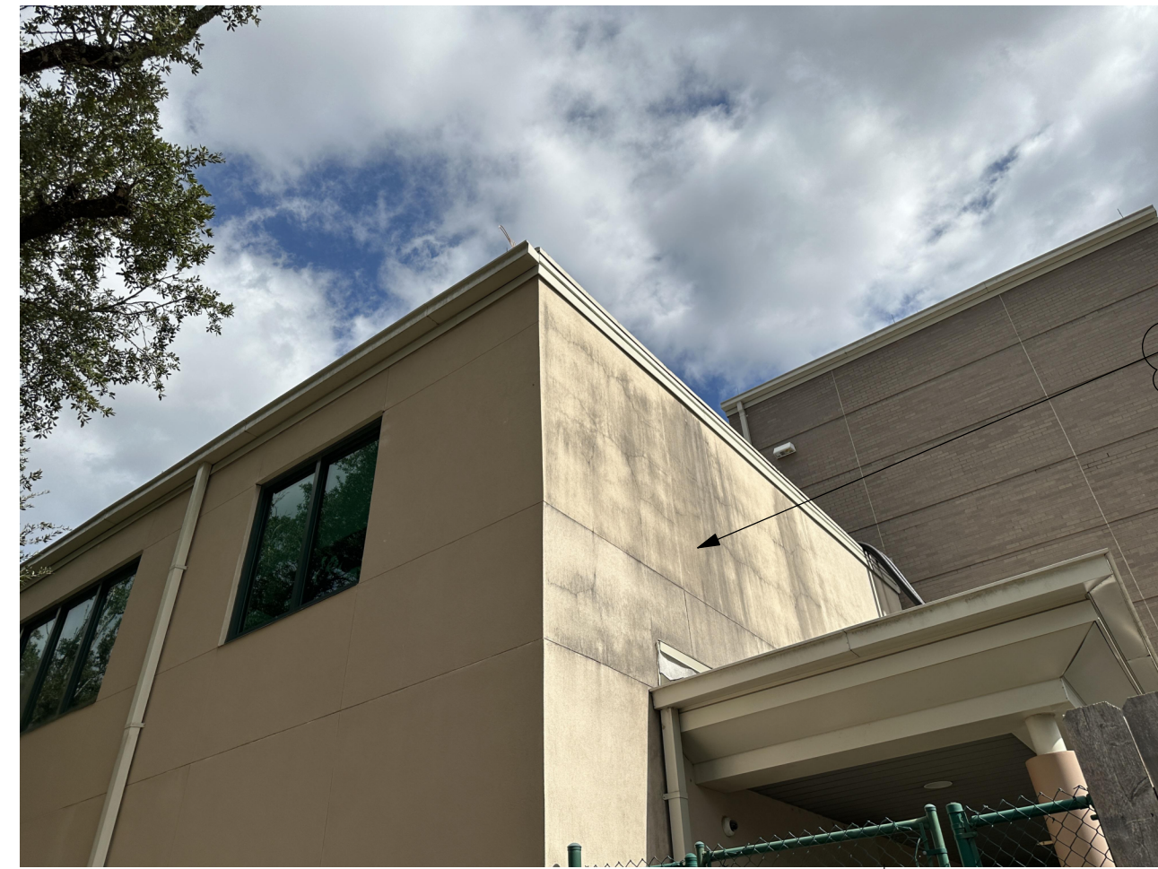
STAINED STUCCO ALONG SIDES OF SINGLE SLOPED ROOFS AT REAR. CLEAN WALL.
