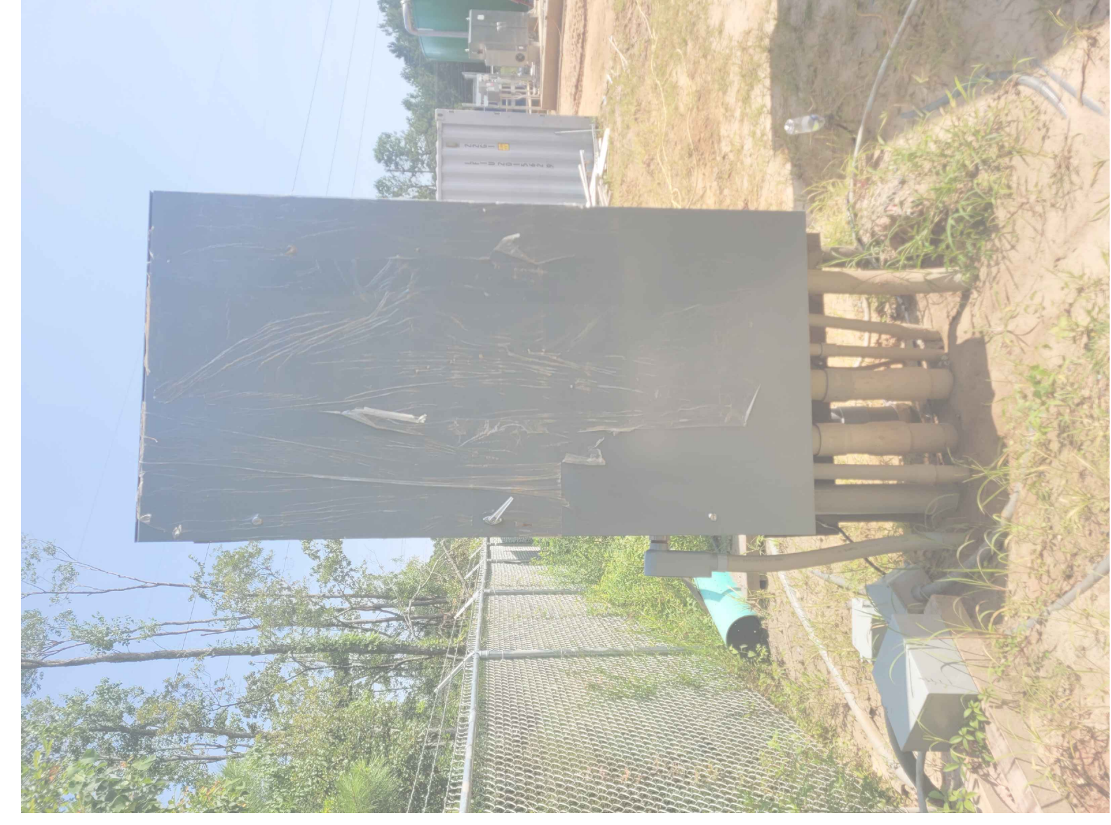
EXISTING PANEL, LOOKING SOUTH
