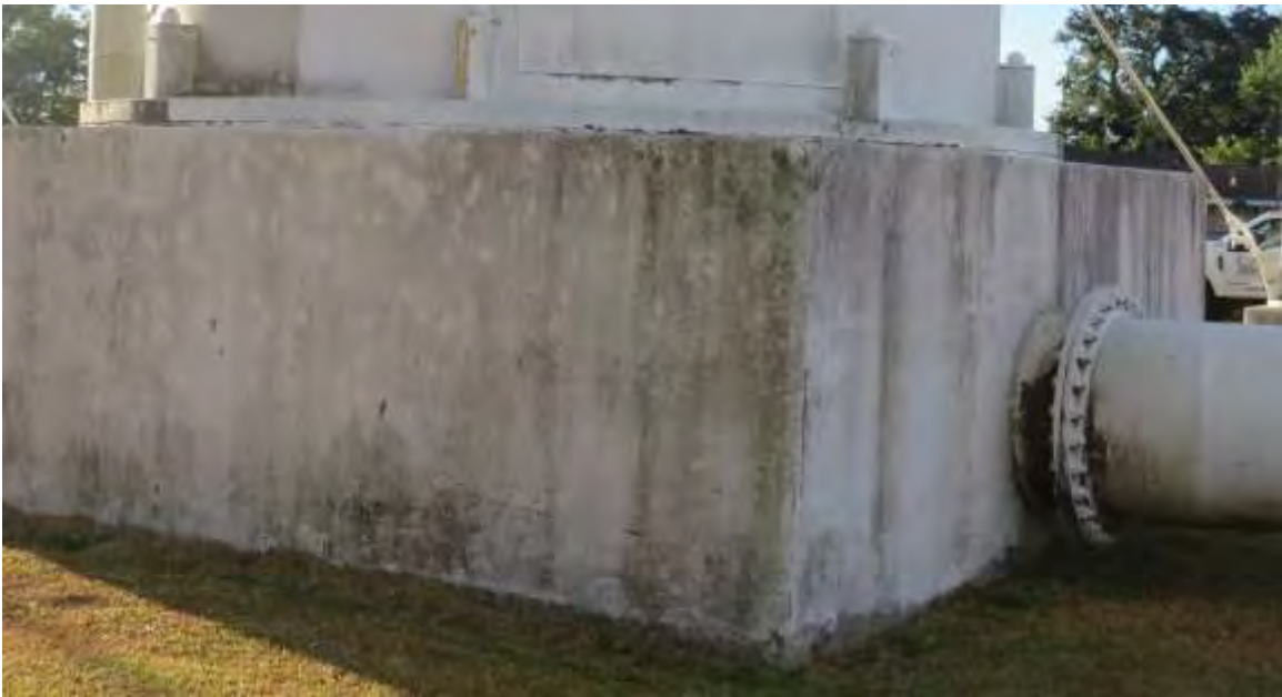
Photos show two (2) examples of the fourteen (14) foundations. We recommend sealing the foundations with a sealant.
