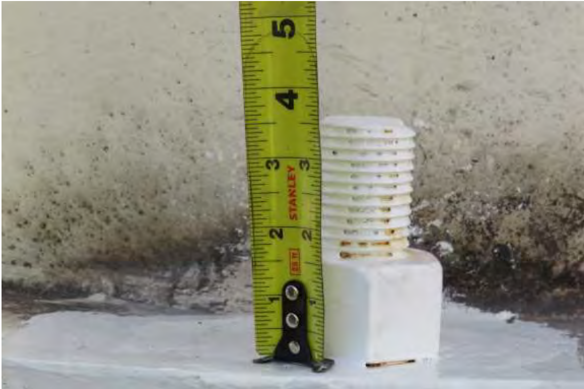
Photo shows one (1) of the anchor bolts, which appear to be in good condition.
