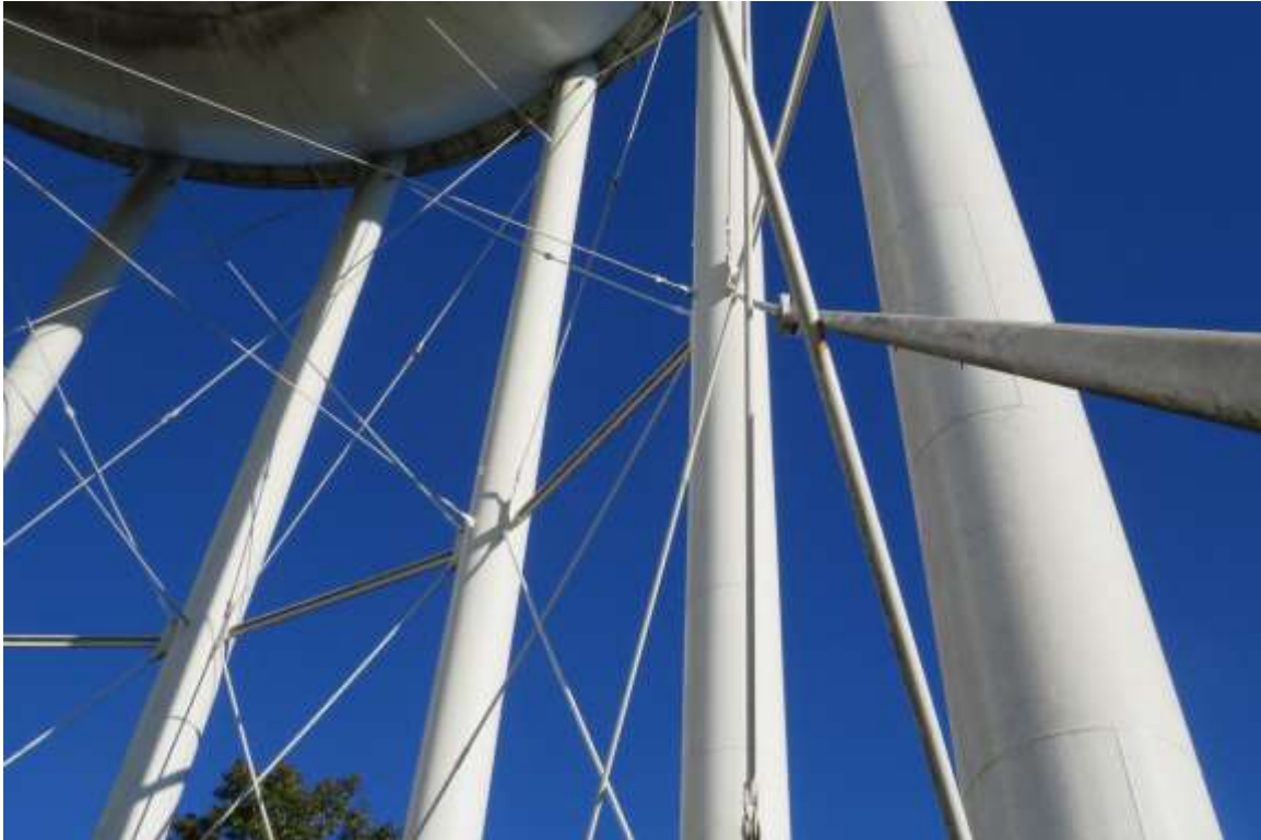
Photo shows the condition of the windage rods, which appear to be in tune and properly adjusted.
