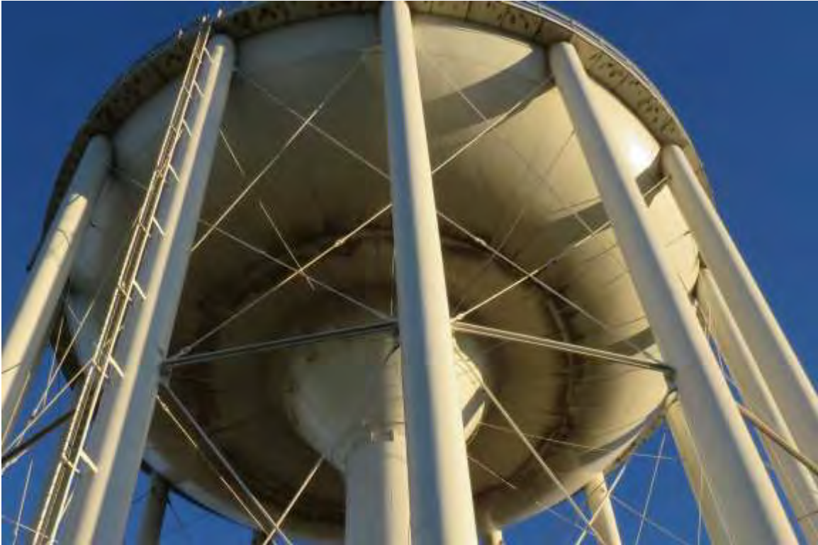
Photo shows the riser pipe and bowl connection, which appears to be in good condition.
