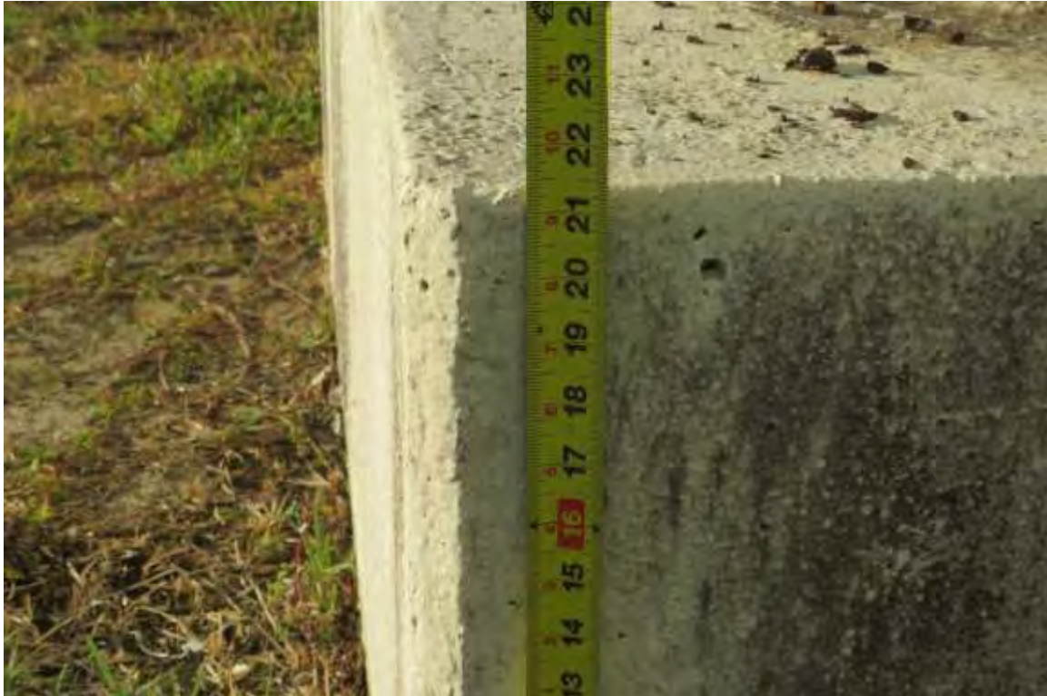
Photo shows the tank foundations are properly graded and in compliance with AWWA D100-21; 12.7.1 Height aboveground.
