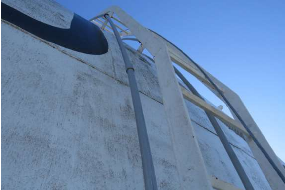
Shell-to-knuckle roof access ladder in above photo is 16” wide in compliance with OSHA 1910.23 Ladders and AWWA D100-21; 5.4.2 Ladders .
