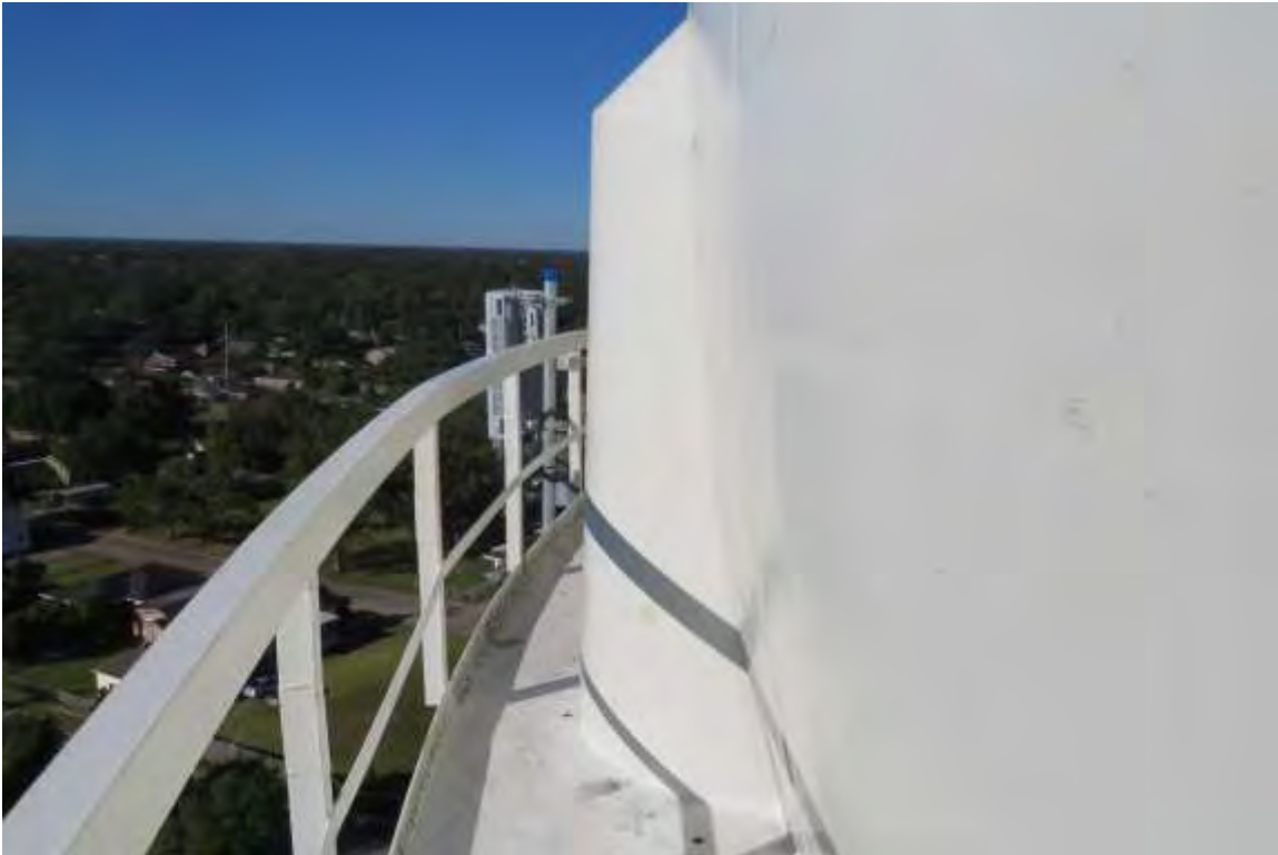
Photo shows the posthead connections. The postheads secure the column legs to the tank shell and support the tank's live and dead load. The postheads have been welded around the circumference of the posthead-to-shell connections for reinforcement and appear to be in good condition.
