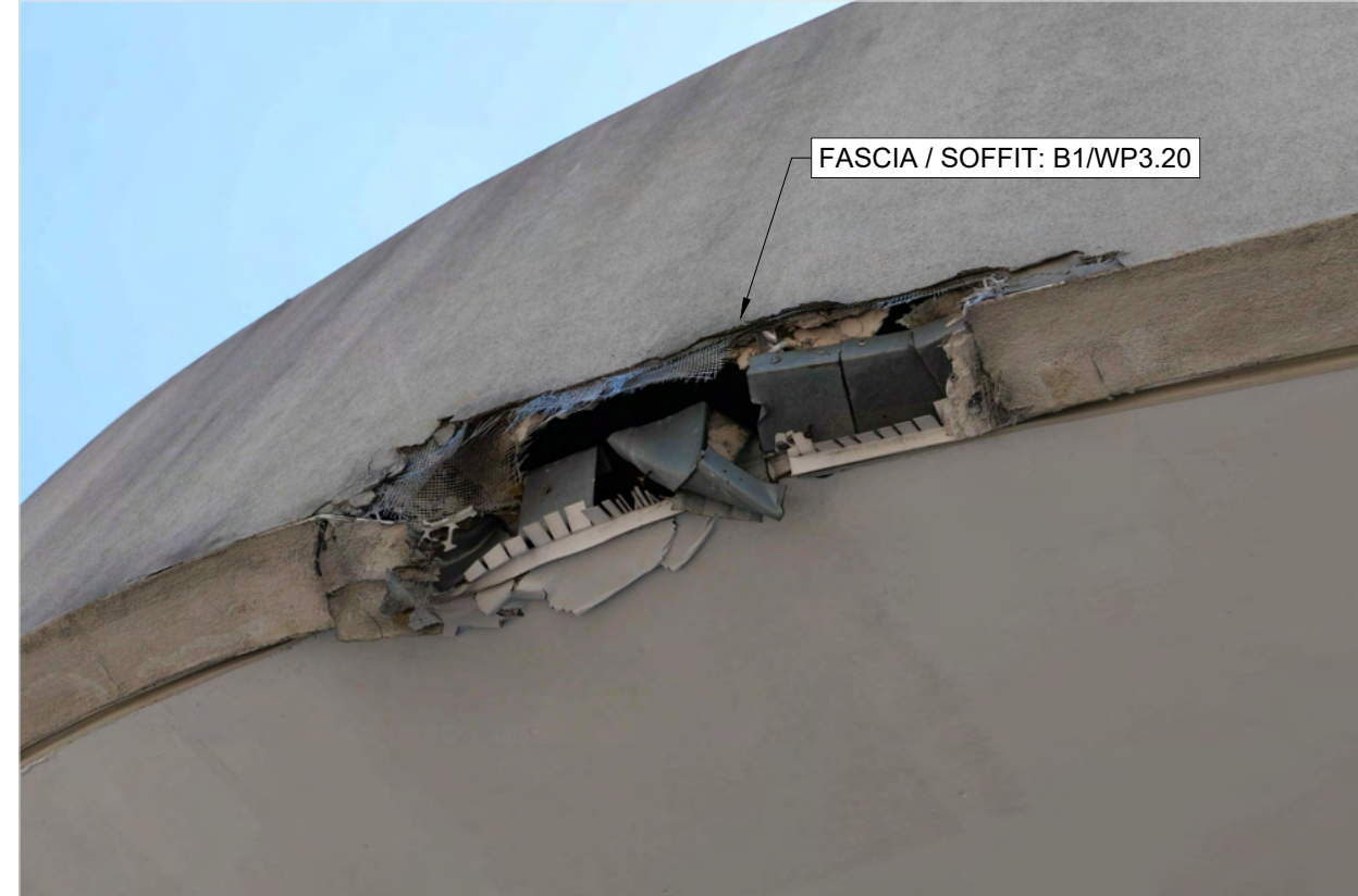
C4 DAMAGED EIFS FASCIA BROW G0.02 SCALE: NONE ARCH REF: NONE
