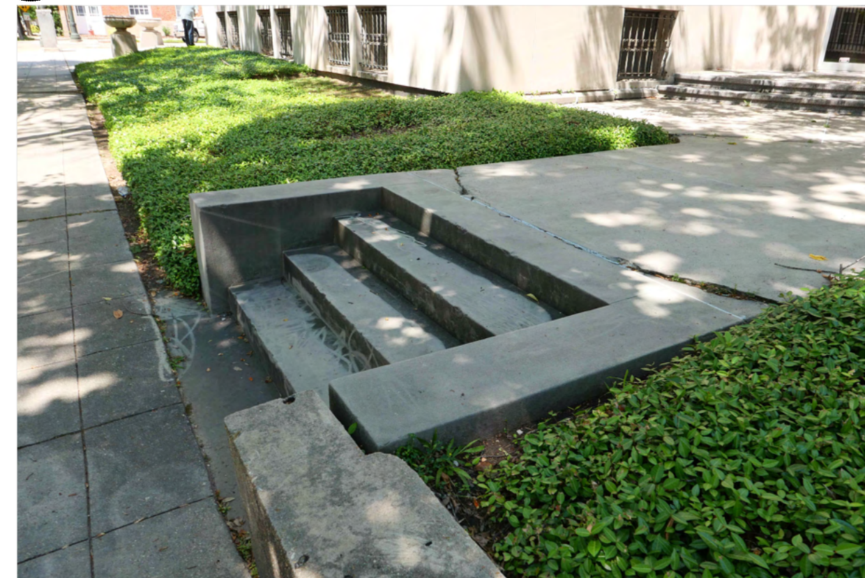
D2 CRACKED AND SHIFTING RETAINING WALL AND SLAB G0.02 SCALE: NONE ARCH REF: NONE
