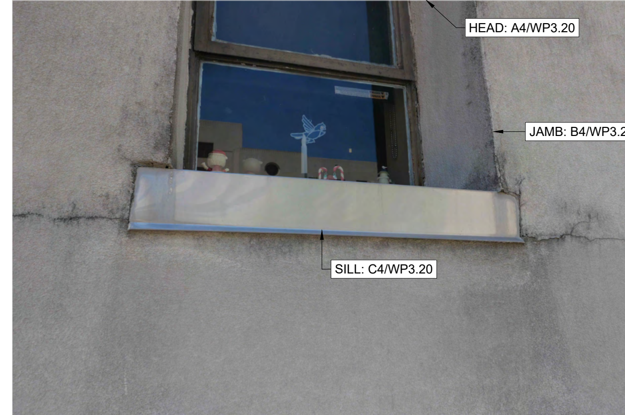
C2 SILL FLASHING AT WINDOW IN EIFS WALL G0.02 SCALE: NONE ARCH REF: NONE
