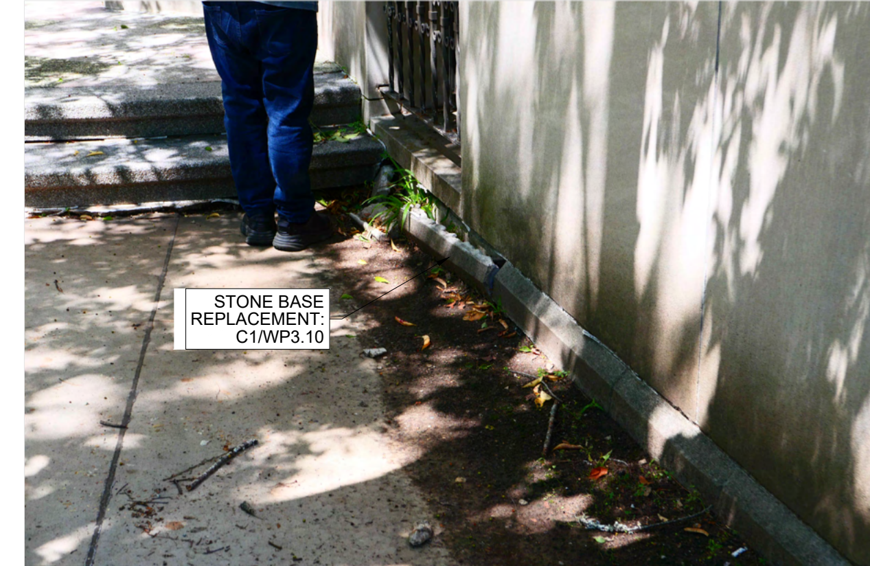
C1 STONE WALL BASE TO BE REPLACED G0.02 SCALE: NONE ARCH REF: NONE
