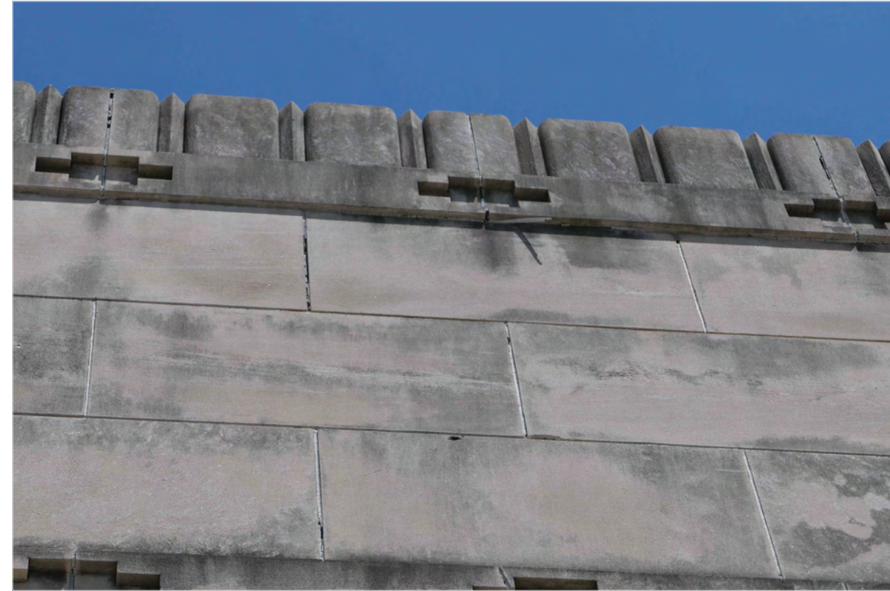
B4 FAILED JOINTS AT TP OF WALL G0.02 SCALE: NONE ARCH REF: NONE
