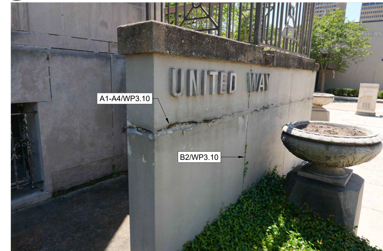
D1 SPALLING AT STUCCO COATED CONCRETE WALL G0.02 SCALE: NONE ARCH REF: NONE
