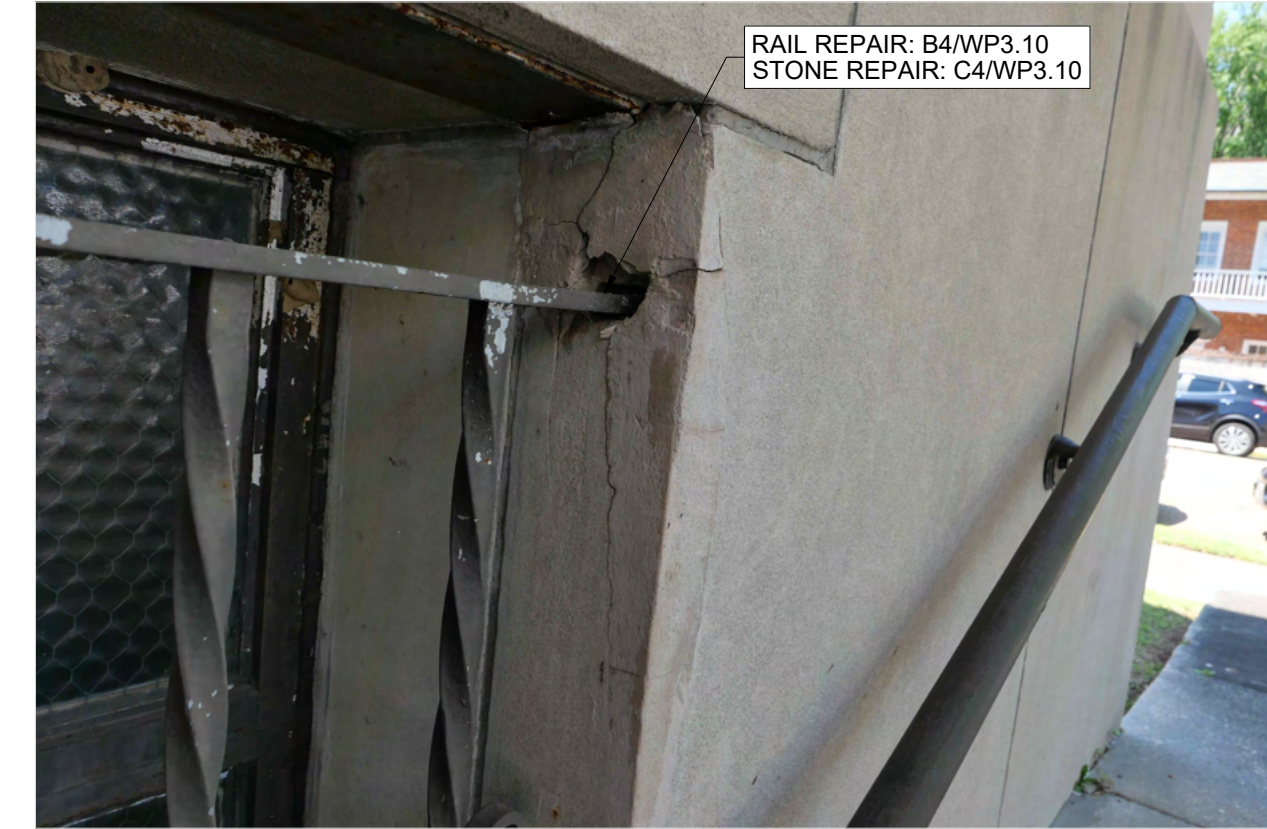
B1 RAILING / CRACKED PANEL G0.02 SCALE: NONE ARCH REF: NONE
