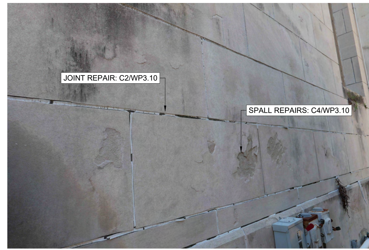
A2 JOINTS TO REPLACE / SURFACE SPALLING G0.02 SCALE: NONE ARCH REF: NONE
