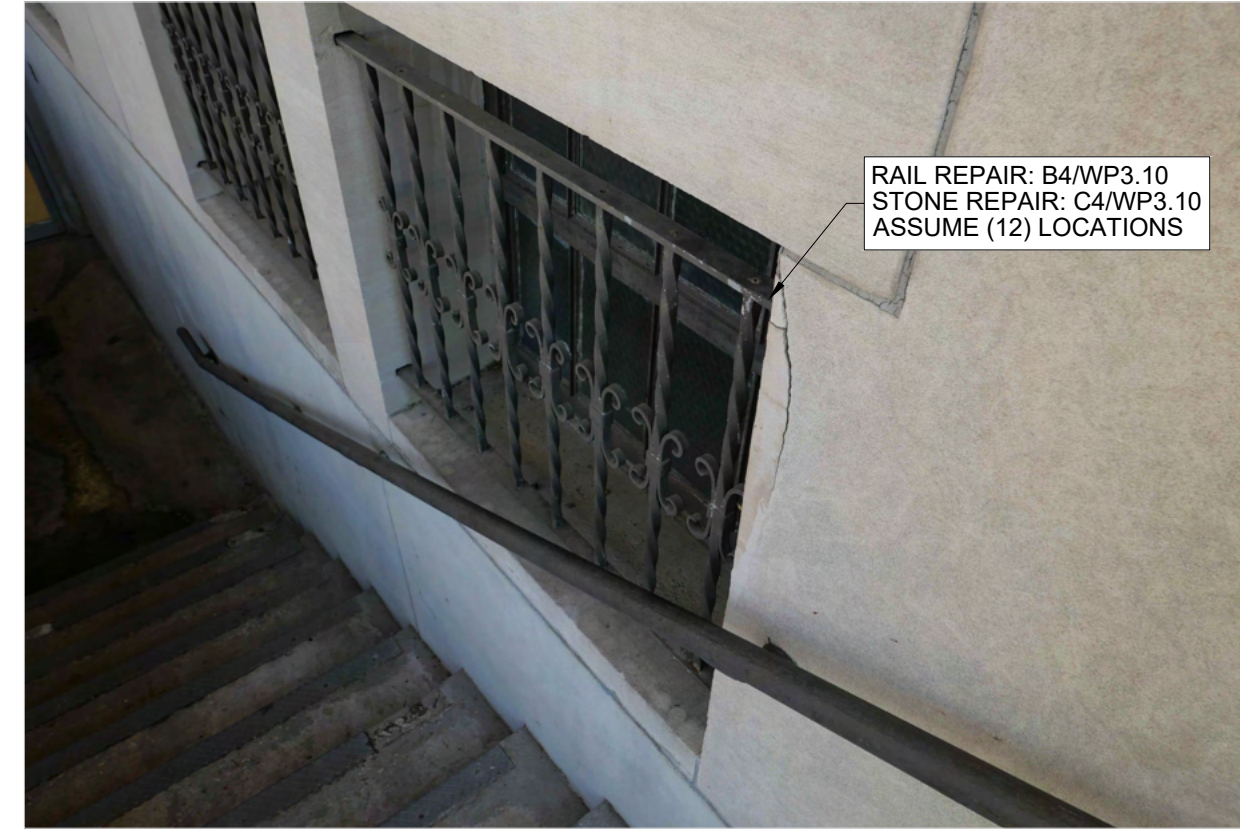
B2 RAILING / CRACKED PANEL G0.02 SCALE: NONE ARCH REF: NONE
