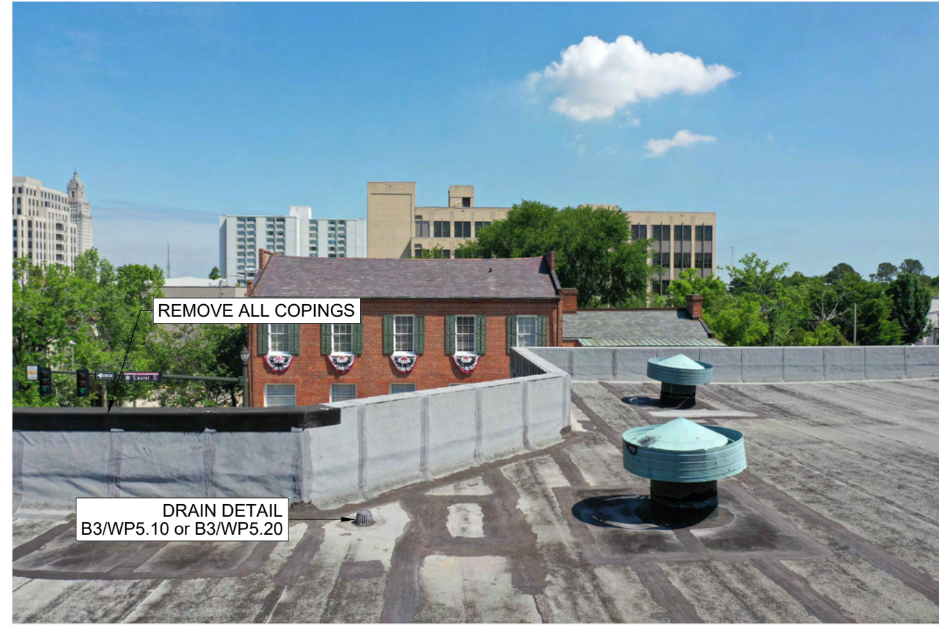
B2 ROOF DRAIN AND ROOF VENT G0.01 SCALE: NONE ARCH REF: NONE
