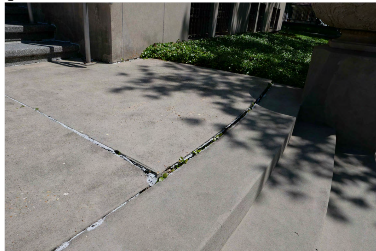
D3 BUCKLED CONCRETE SLAB AT STEPS G0.02 SCALE: NONE ARCH REF: NONE
