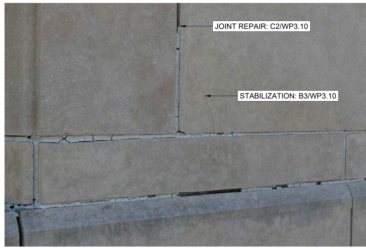
A3 JOINTS TO REPLACE / CRACKED PANEL G0.02 SCALE: NONE ARCH REF: NONE
