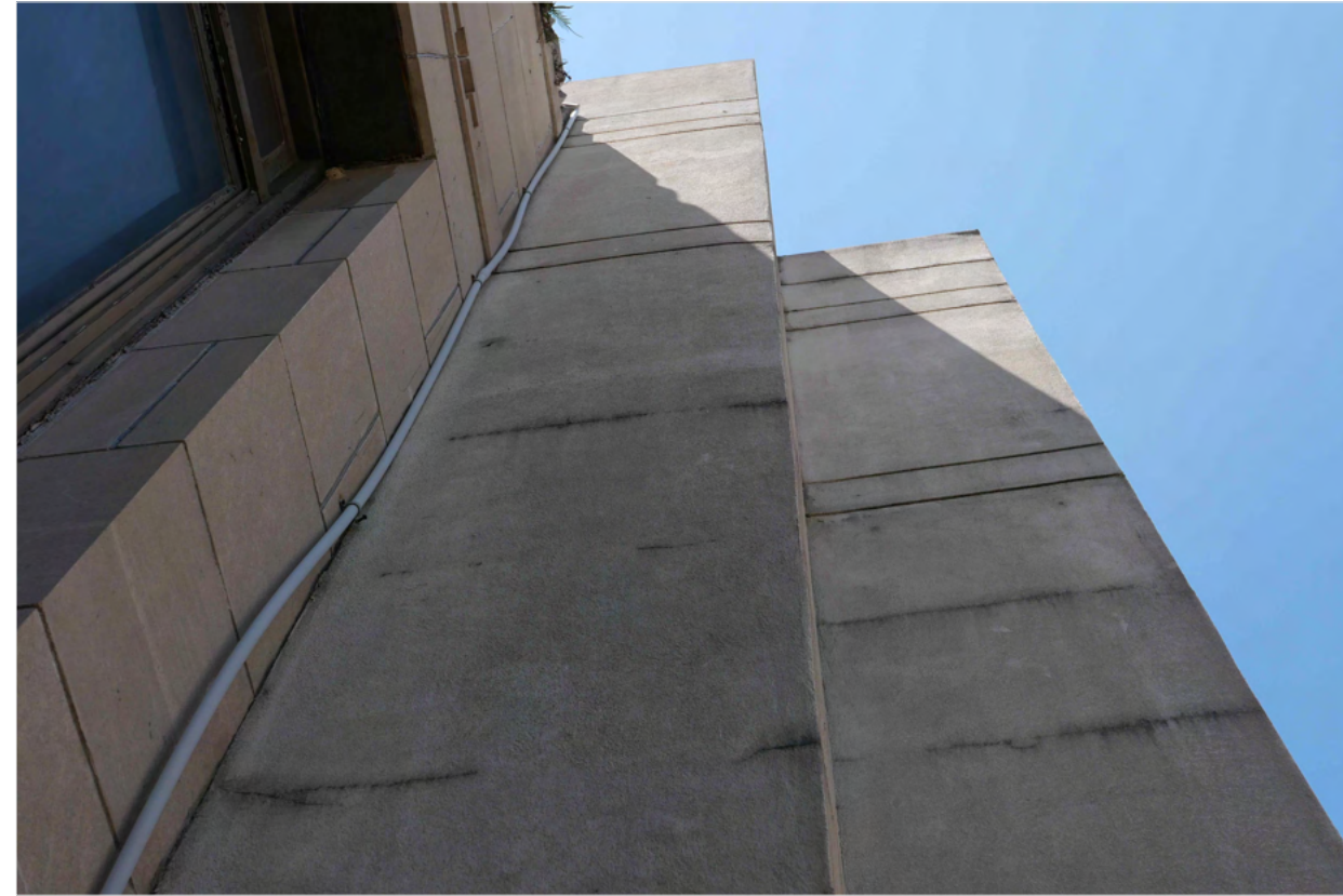
B3 FAILING EIFS ADJOINING STONE PANEL G0.02 SCALE: NONE ARCH REF: NONE
