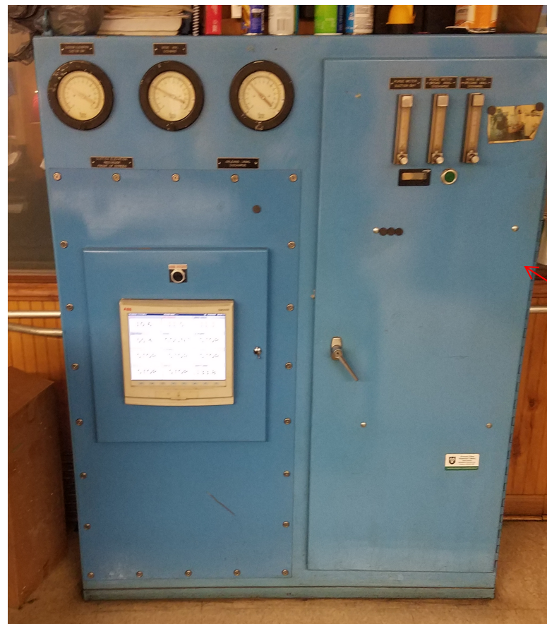
Existing PLC Cabinet - PLC rack located on interior of door.
