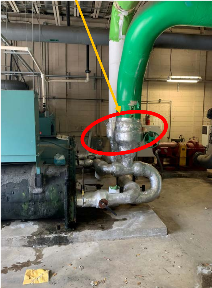
Point #1 for Chilled Water Lines
