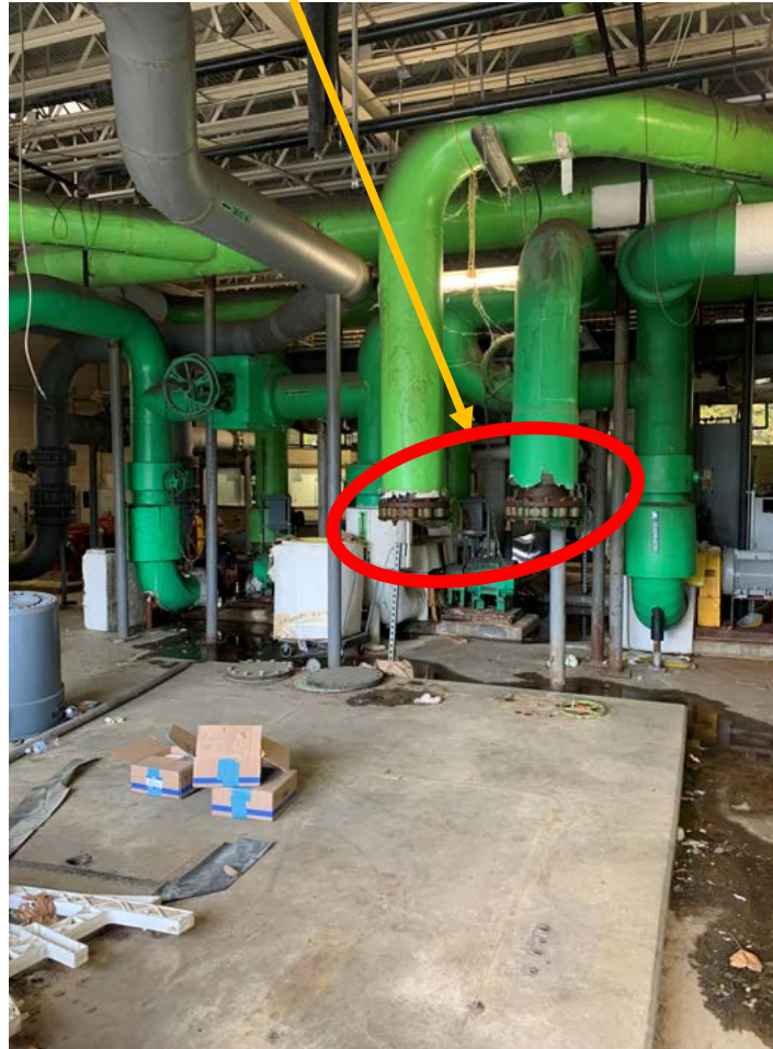
Point #2 for Chilled Water Lines
