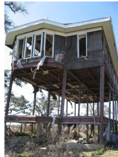
Post-Katrina wind and wave damage in Waveland
